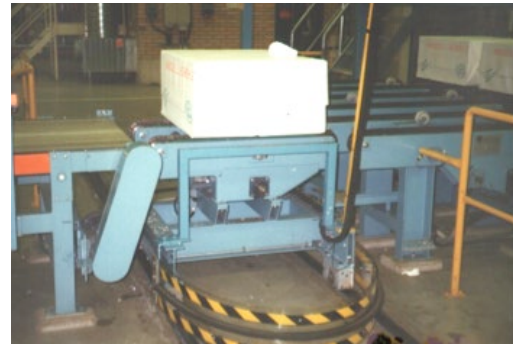
Traveling chain conveyor for single bales.
